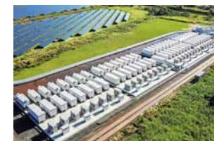
Storage batteries at Suzuran Kushiro cho Solar power plant
