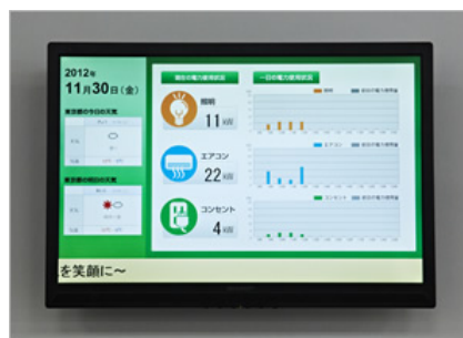
Energy management monitor for each floor
