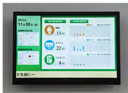
Energy management monitor for each floor
