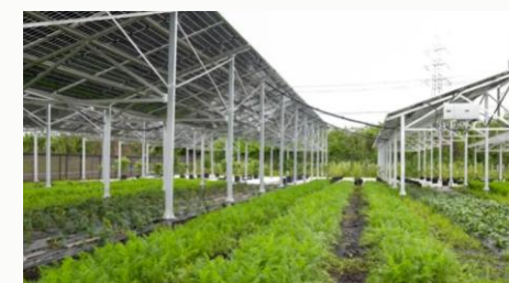
Solar panels and vegetation management beneath them (ReENE Solar Farm Higashimatsuyama)
