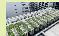
The Unosawa Tokyu Building's potato-based greening system
