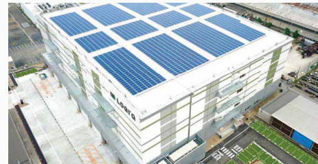
ReENE LOGI'Q Kyoto Kumiyama Solar Power Plant
