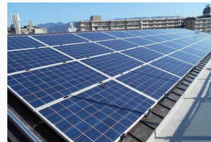
Solar panels on the roof of a condominium complex
