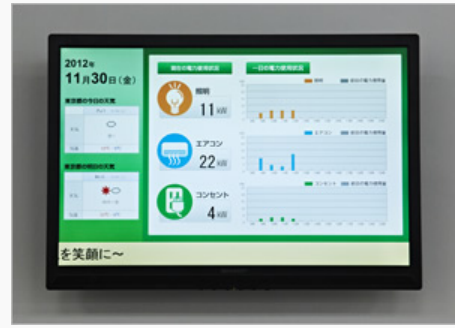
Energy management monitor for each floor
