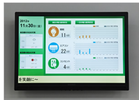
Energy management monitor for each floor
