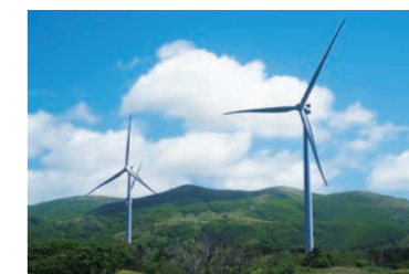
ReENE Matsumae Wind Farm (Commencement of operation: April 2019)
