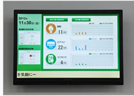
Energy management monitor for each floor
