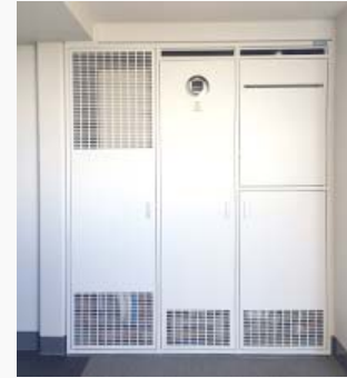
Enefarm for condominiums
