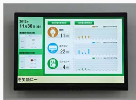
Energy management monitor for each floor
