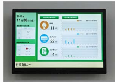
Energy management monitor for each floor
