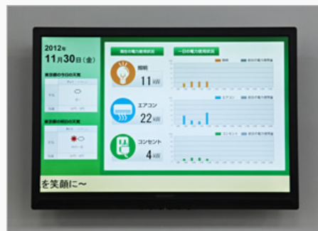
Energy management monitor for each floor
