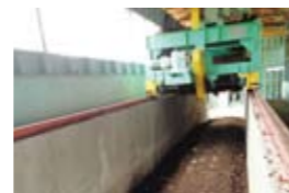
Compost waste disposal facilities
