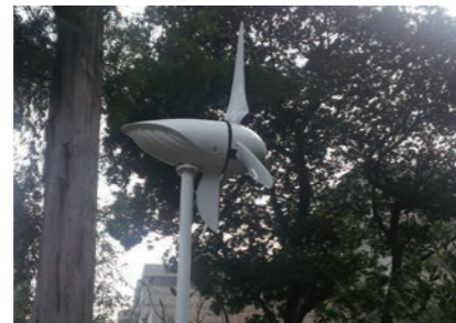
Wind turbine installed within the premises of Tokyu Harvest Club Atami Izusan & VIALA
