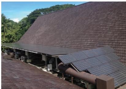
Solar power generation at the Palau Pacific Resort
