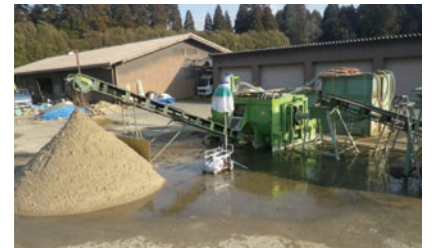
Bunker sand washing system
