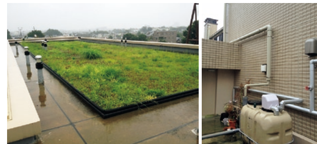
Rain water is collected on the roof for watering the garden.
