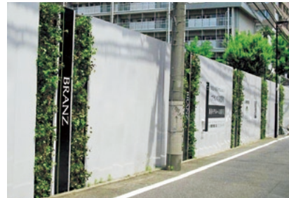
Temporary enclosure with greenery (BRANZ Yonbancho)
