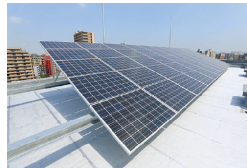
Solar panels for solar power generation of "BRANZ Higashi Ikebukuro"
